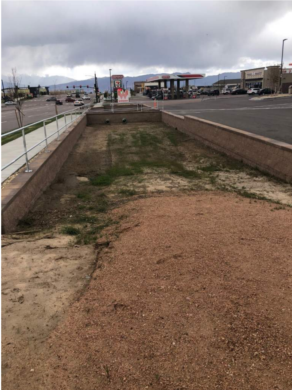
Overall Site / Infiltration Media (East forebay)
